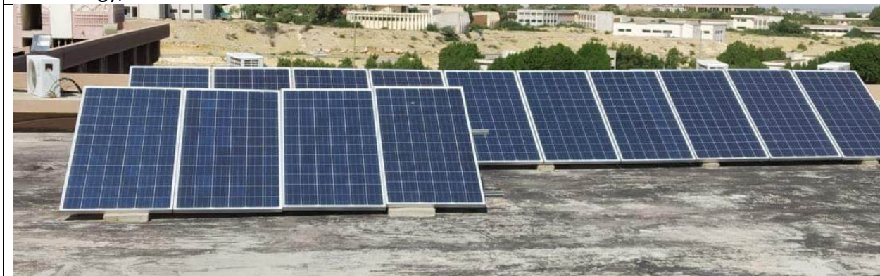
Solar Panels installed at Main Administration Building of Mehran University of Engineering & Technology, Jamshoro
