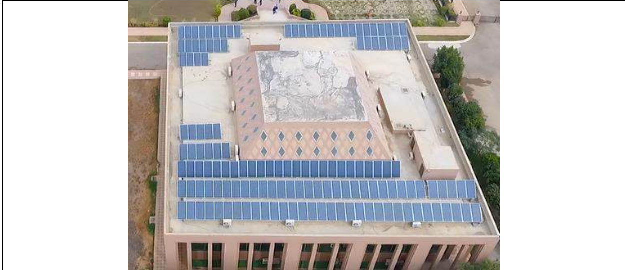
Solar Panels installed at Central Library Building of Mehran University of Engineering & Technology, Jamshoro
